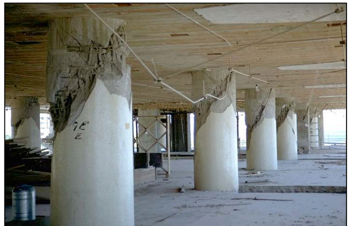
Earthquake damaged structure
