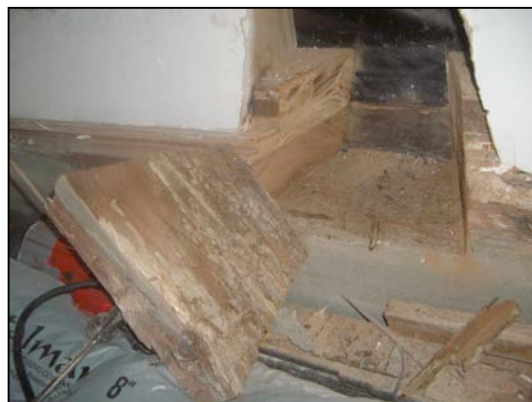
Example of wood rot
